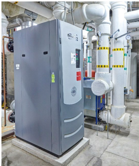
A large condensing boiler provides primary heat for the building's IPS fan coil system.
