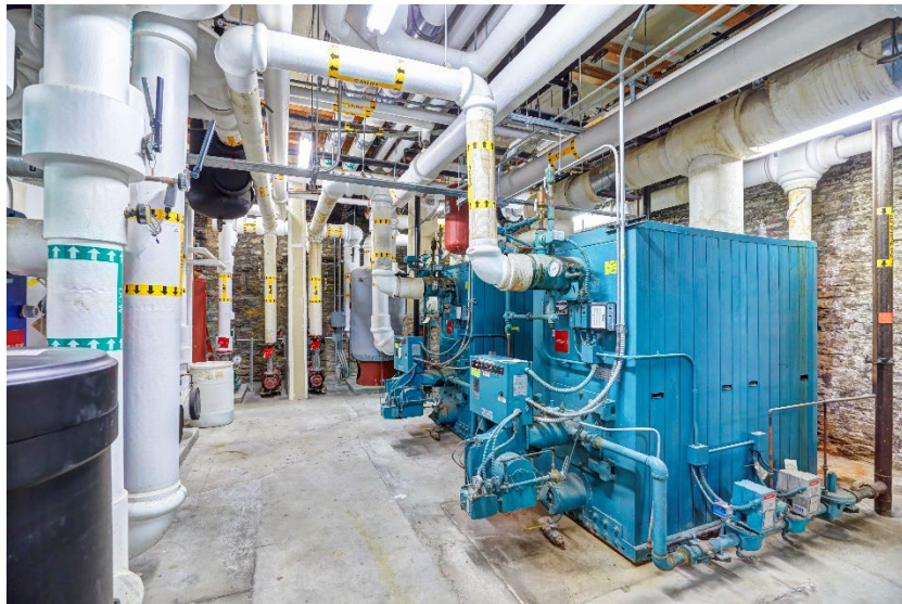
Two redundant atmospheric boilers provide supplementary heat for the building's IPS fan coil system.
