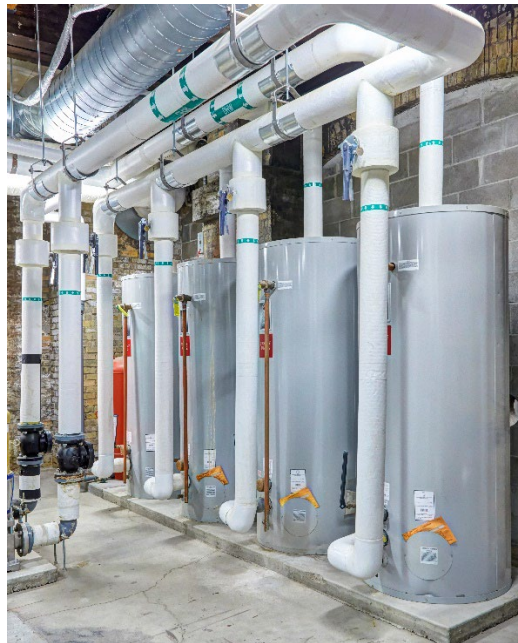
Four, 200-gallon hot water tanks provide storage for the building's DHW and IPS hydronic systems.
