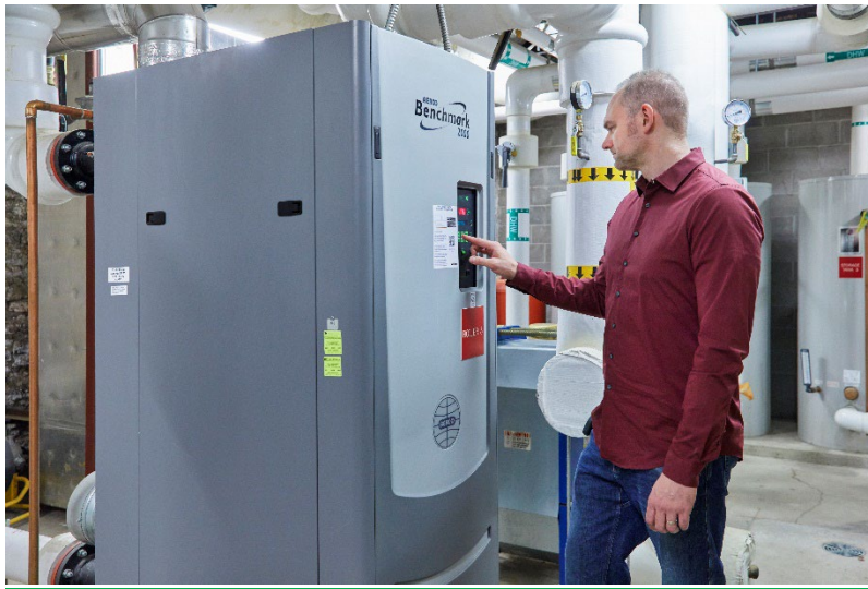
Tom Suek, director of facilities at Hewing Hotel, checks the supply water temperature on the building's primary boiler.
