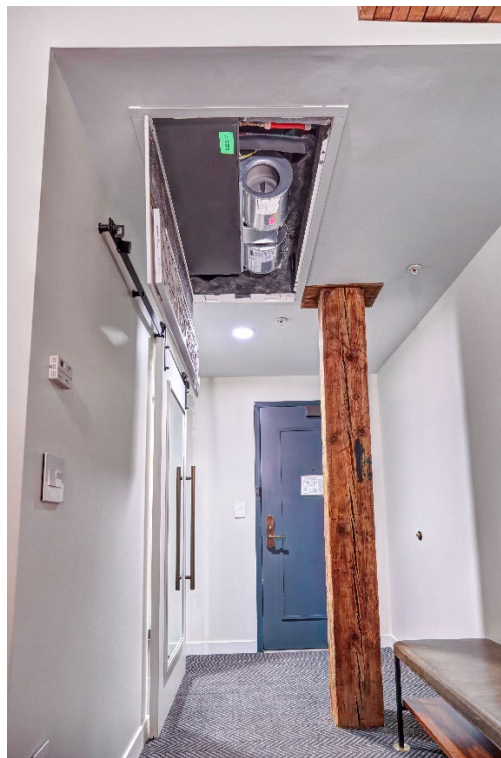
Guest rooms are heated and cooled by a Williams Comfort Products IPS fan coil unit.
