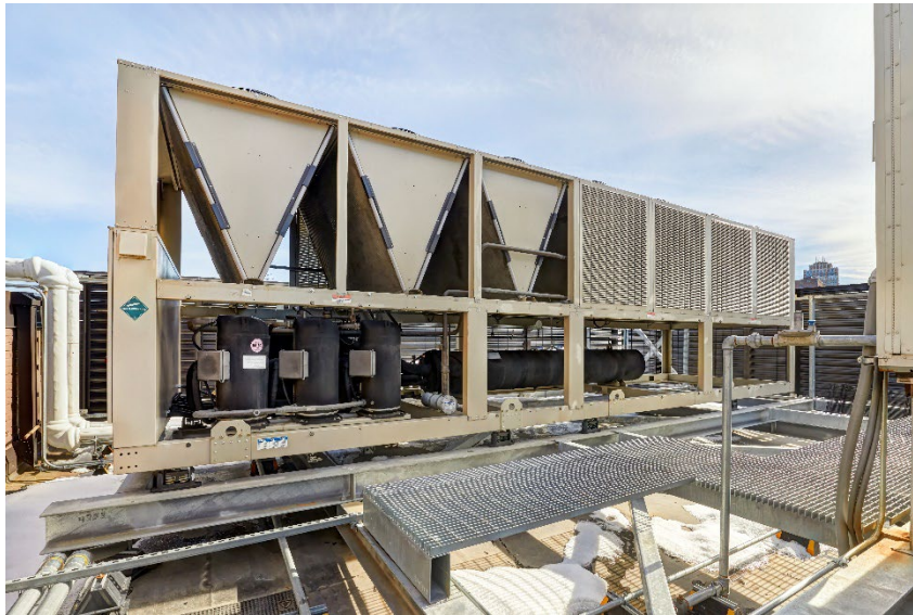
An air-cooled chiller is used to supplement cooling capacity for the IPS system.
