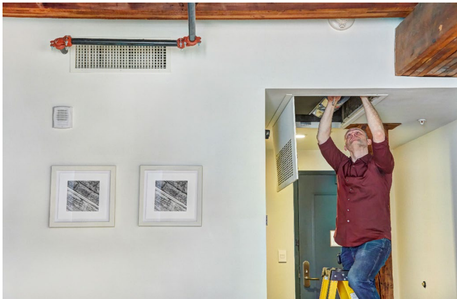
Tom Suek, director of facilities at Hewing Hotel, checks a Williams Comfort Products IPS fan coil unit in one of the 124 guest rooms.
