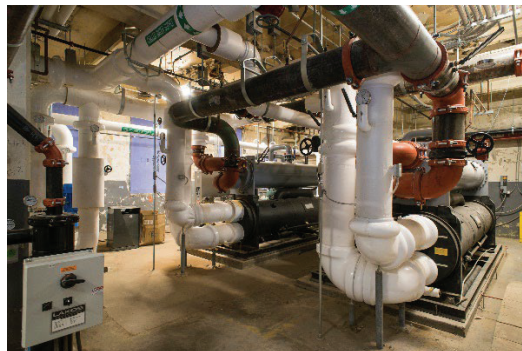
A pair of 375-ton Dunham Bush screw compressors provide supplementary cooling capacity only when economizer cooling is not enough to satisfy the building's cooling load.
