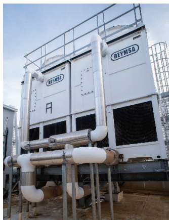
The fiberglass cooling tower used to provide supplementary cooling capacity for The Atlantic's IPS hydronic heating and cooling system.
